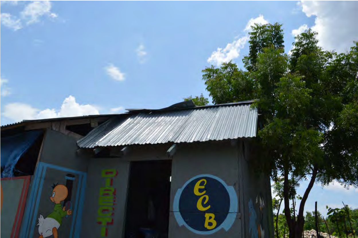
Parts of roof falling off
