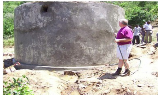
Charlie Lyddane, a member of the Rotary Club of West Chester, hoses down the sides of a new water tank in Nuu Kenya to seal the exterior.
