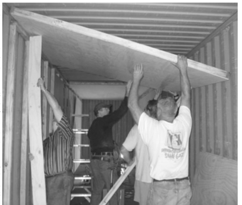
Volunteer workers install the ceiling in the container which will become the water filtration plant for Jos Nigeria.
